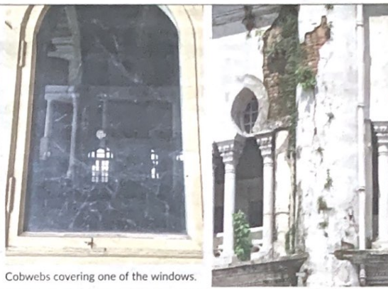
Cobwebs covering one of the windows.
