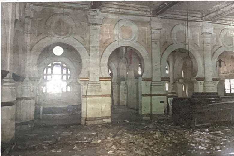
Heritage Hotel, located within the Kuala Lumpur train station, is in dismal state.
