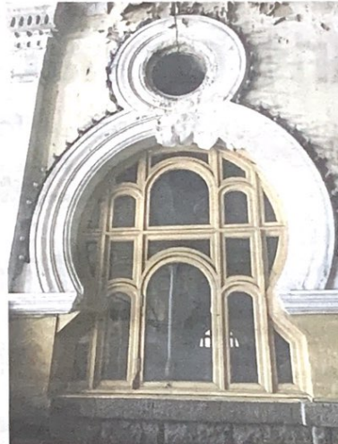
Peeling paint on the walls of the Kuala Lumpur train station is obvious.
